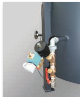
■ Cooling water inlet group
